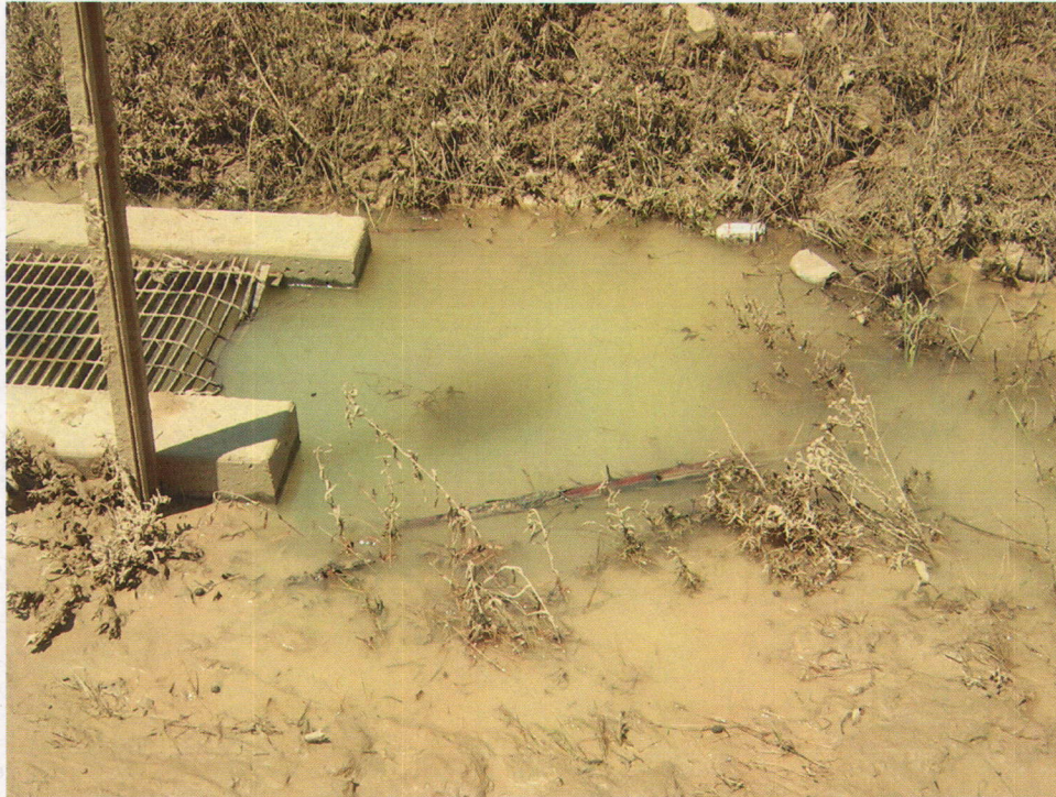
Photo No. 7 – The stagnant water surrounding the County constructed culvert was visually observed to be opaque and high in total suspended solids. The dump material matted nearby vegetation but the vegetation was still not uprooted.
