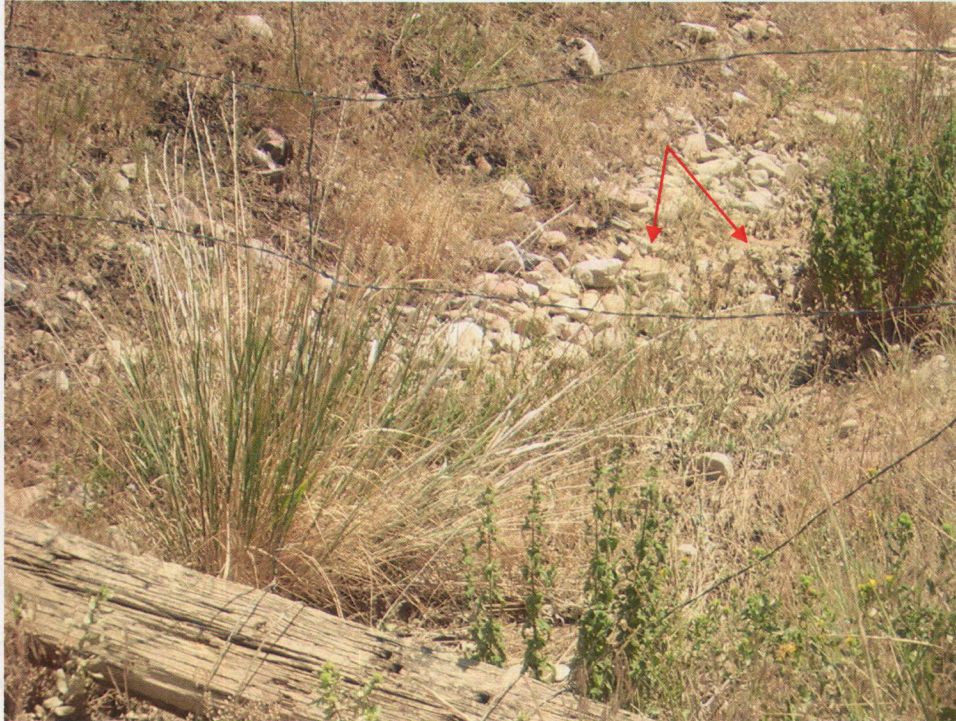
Photo No. 13 – Pictured is the County constructed drainage channel just below the outlet structure for the culvert. Note the established vegetation and intact riprap. Also note the limited distribution of dump material (coffee color) located between the rocks comprising the riprap cover (red arrows).
