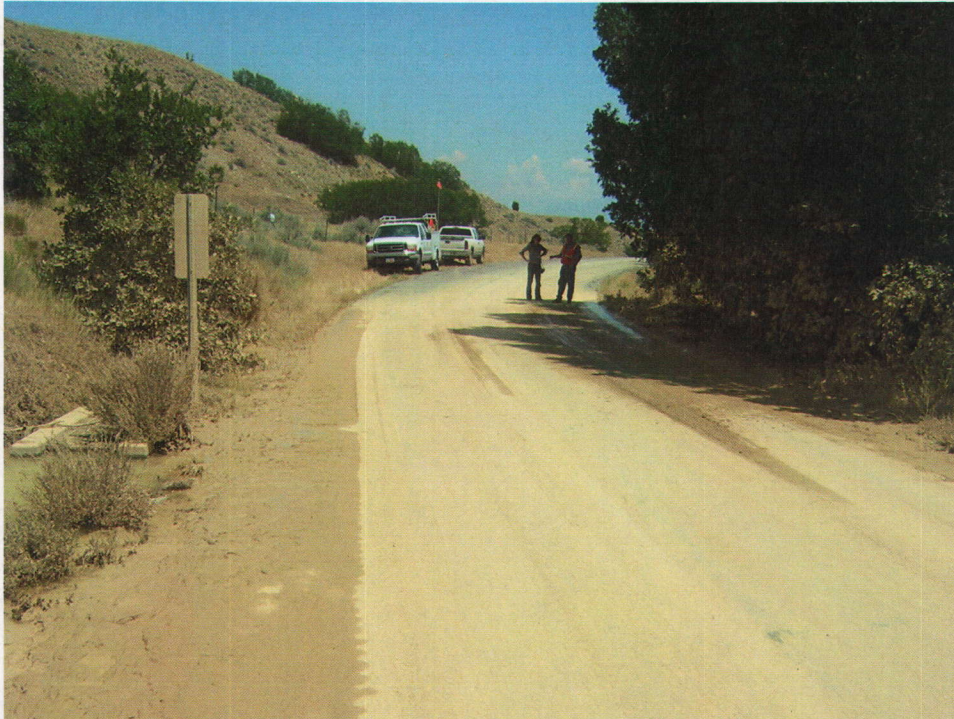
Photo No. 5 – Pictured is a lower (in elevation) section of the County Road in Butterfield Canyon, where because of a blockage in the underlying culvert (inlet pictured to the forefront of the street sign) the runoff flow (storm water / dump material) from Yosemite Drainage crossed to the south side of the County Road and into the County constructed drainage channel to Butterfield Creek. The two persons in the shadow of the trees are Ms. Peacy and Mr. Vinton. Note the stagnant water surrounding the inlet to the County constructed culvert.
