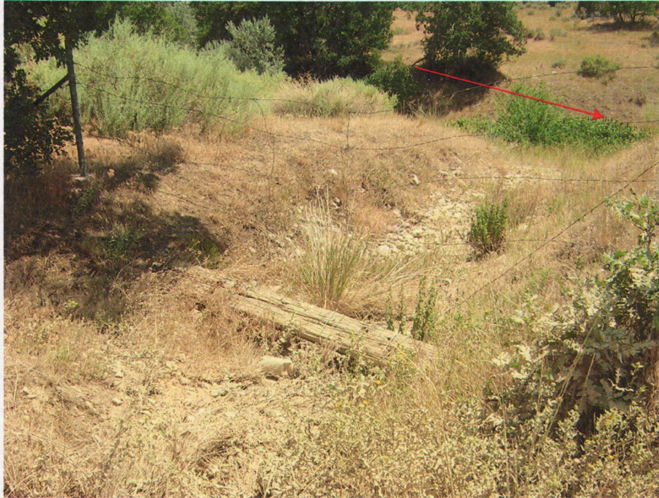
Photo No. 11 – Pictured is the County constructed drainage channel leading from the outlet of the County constructed culvert underlying the County Road in Butterfield Canyon. The outlet for the culvert was (when pictured) buried. The vegetation in the channel appeared to be relatively intact, with some matting due to deposited dump material. The riprap in the lower section of this channel also appeared to be intact. Butterfield Creek channel is denoted by the red arrow.
