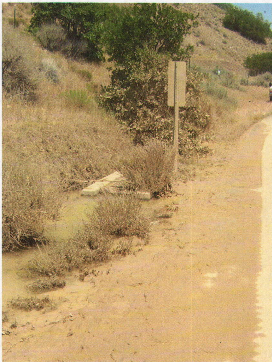
Photo No. 6 – Pictured is the north side of the County Road and the County constructed culvert inlet. Note the stagnant water and dump material deposited along the side of the road.
