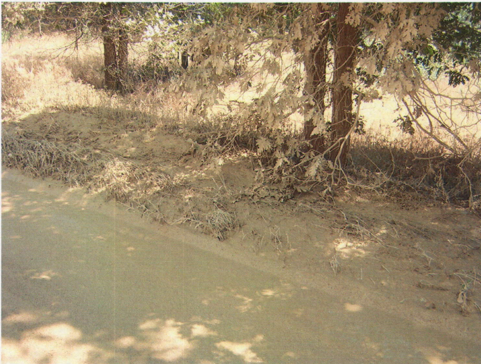
Photo No. 10 – From the same vantage point as Photo No. 9 (but looking southeast from the County Road), one can view the distribution of dump material. Note that even though matted significantly, the vegetation along the south side of the road (grasses predominantly) were not uprooted.
