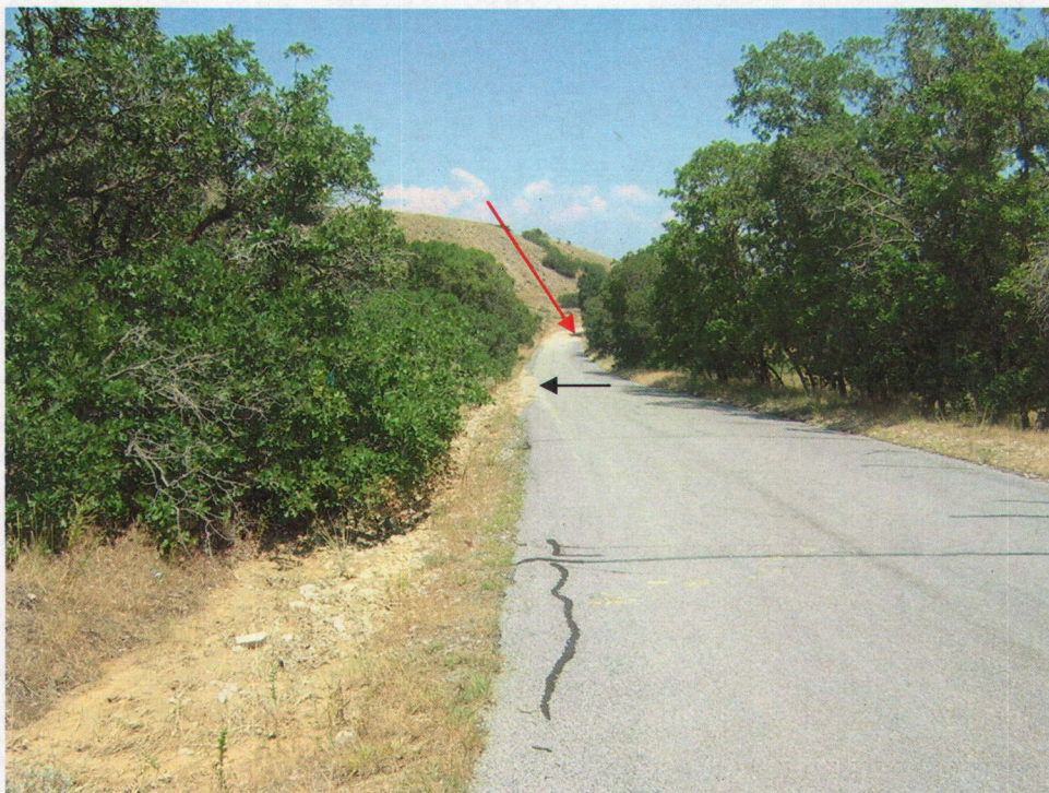
Photo No. 4 – Pictured is the County Road viewed from the lower section of Yosemite Drainage. The Black arrow points out a location where runoff material skirted onto the road surface. The Red arrow points out the location (approximately 300 feet to the east) that the runoff flow (storm water / dump material) crossed the County Road. Note that for the most part the runoff was contained to the north side of the County Road.
